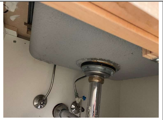
Photo 6: HM-E: Sink Insulation, Gray
