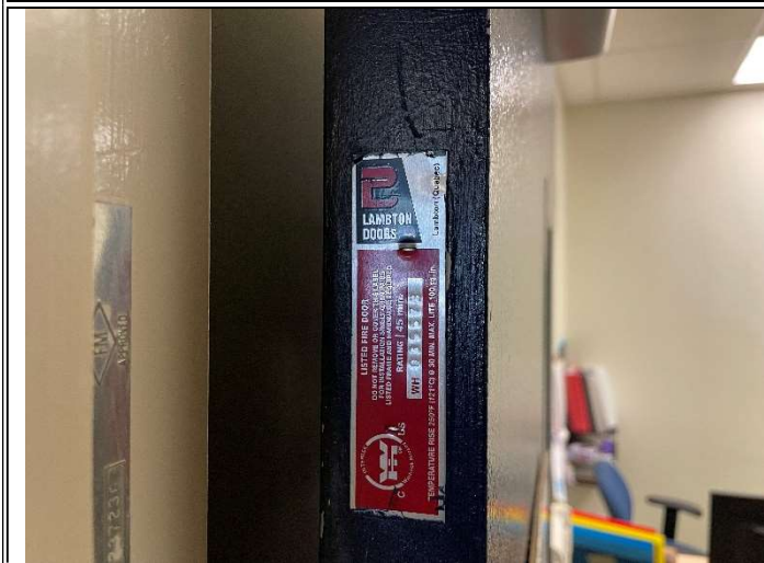
Photo 11: HM-J: Fire-rated Door Insulation, Red Tag with Silver Lettering
